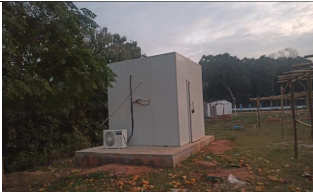
Fig: Cold storage
