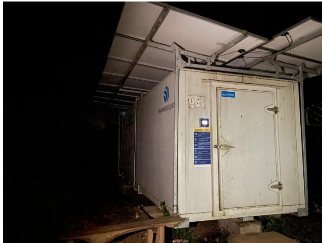
Fig: Cold storage
